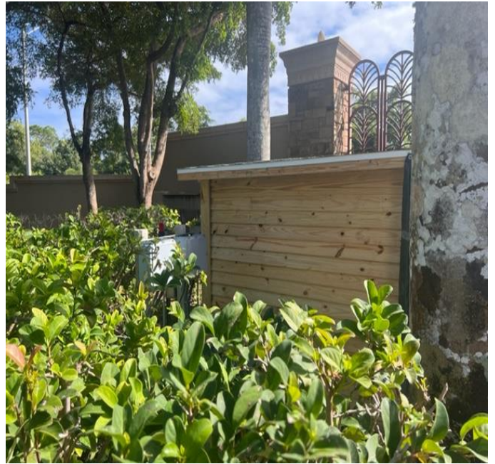
The newly installed above ground irrigation pump house located on the west side of the main entrance.
