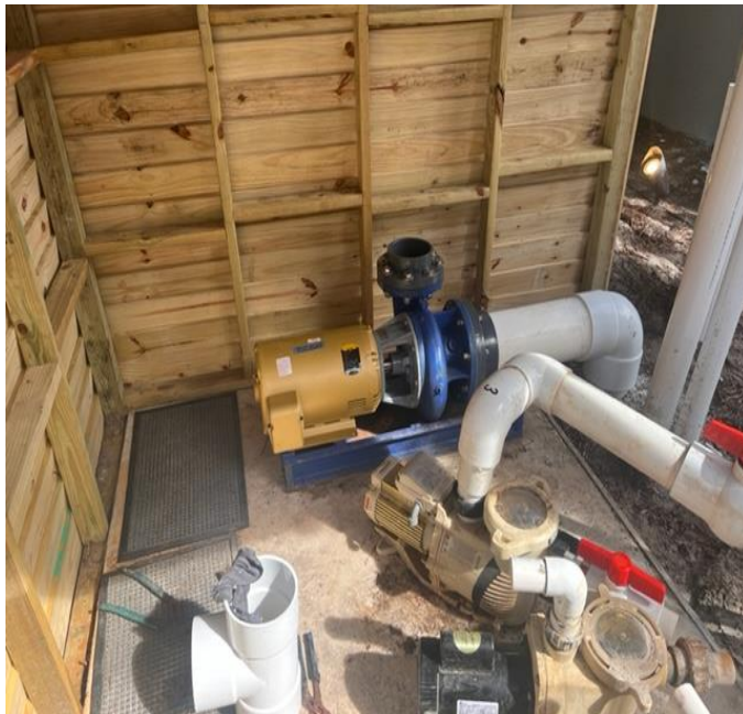
Newly installed 15 HP pump located in the pump house on the west side of the main entrance.
