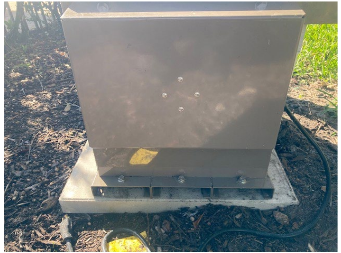
Lake 7 aeration box set-up
