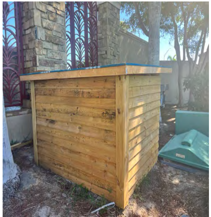
NEW ABOVE GROUND PUMP HOUSE
