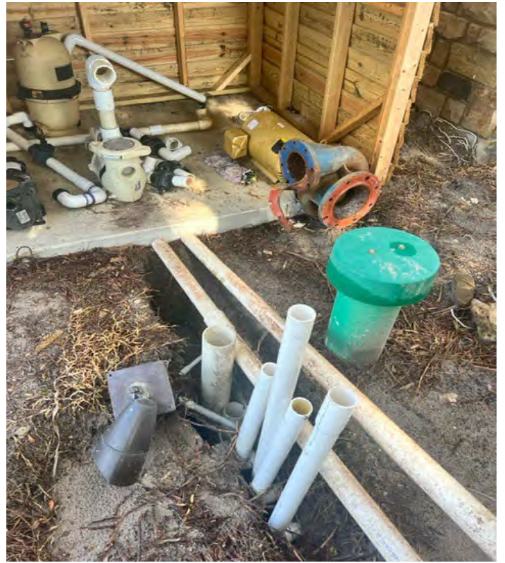
EAST POOL FOUNTAIN PLUMBING
