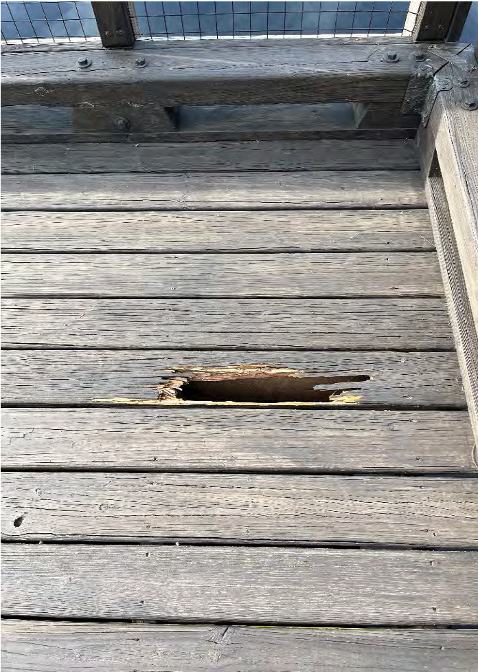
Hole in the wood on boardwalk
