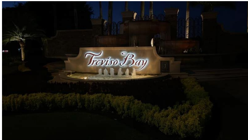
Entrance monument sign and fountain with new backlighting.
