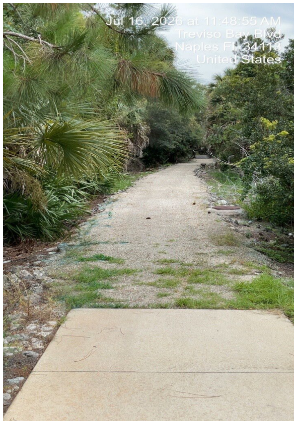
Walking Trail that needs attention
