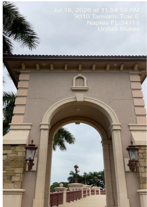
Tower Soffit Lighting
