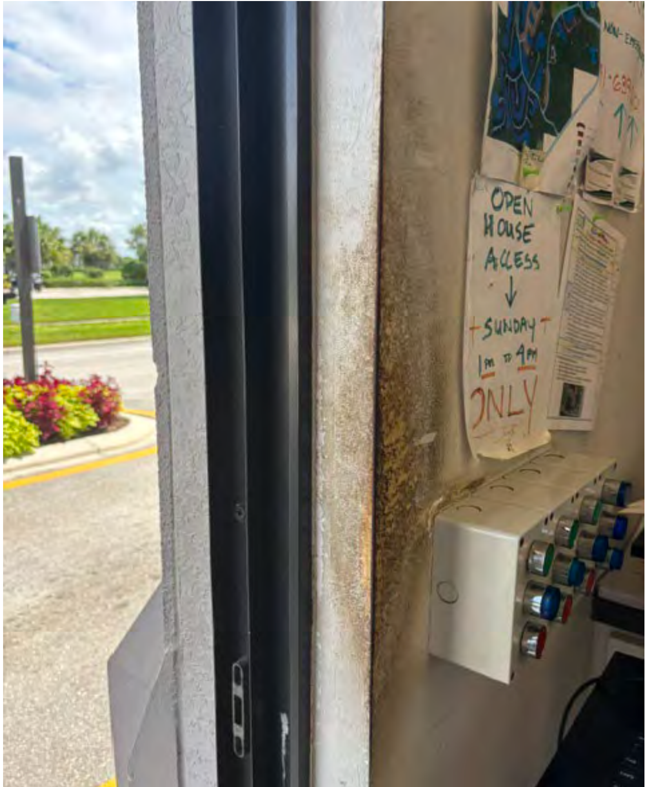
Need guard handrail (currently untouchable and missing)
