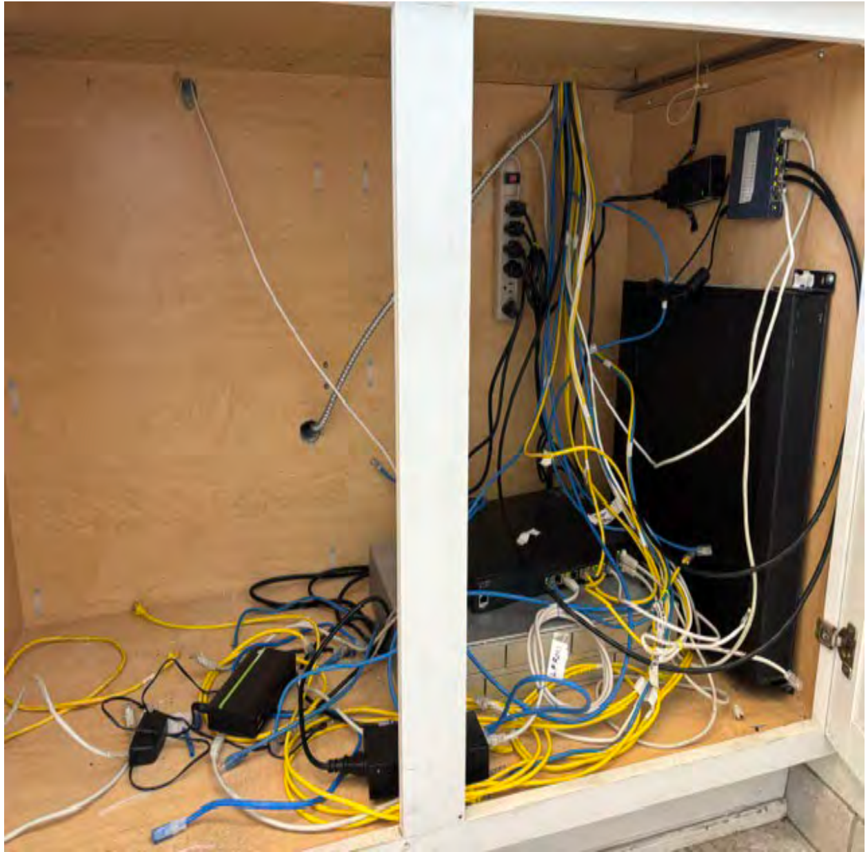
Camera equipment in cabinet
