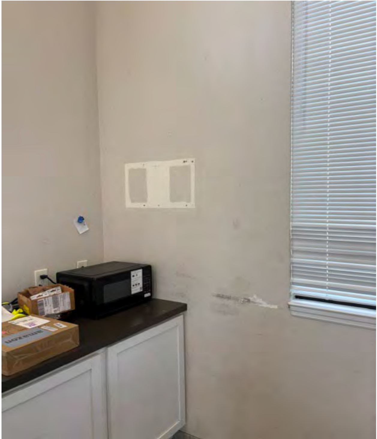
Visible wall that shows interior needs to be painted
