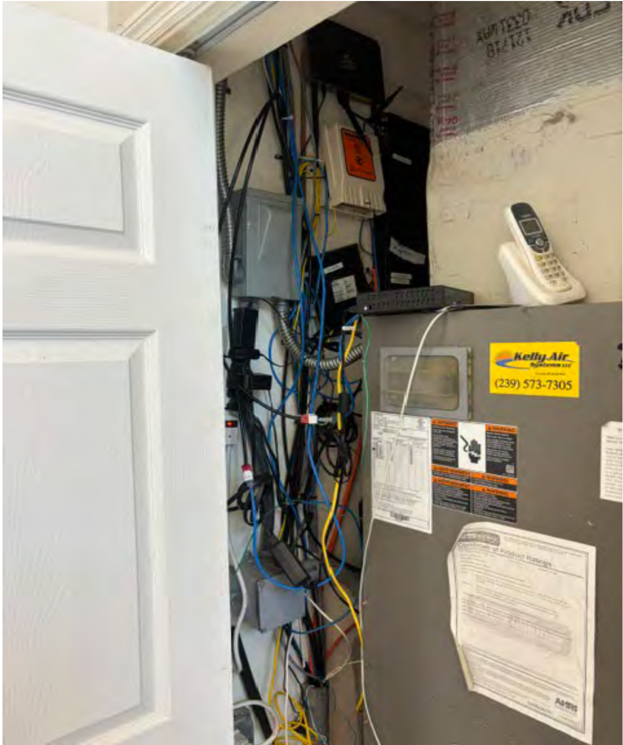
Modem and equipment in HVAC closet
