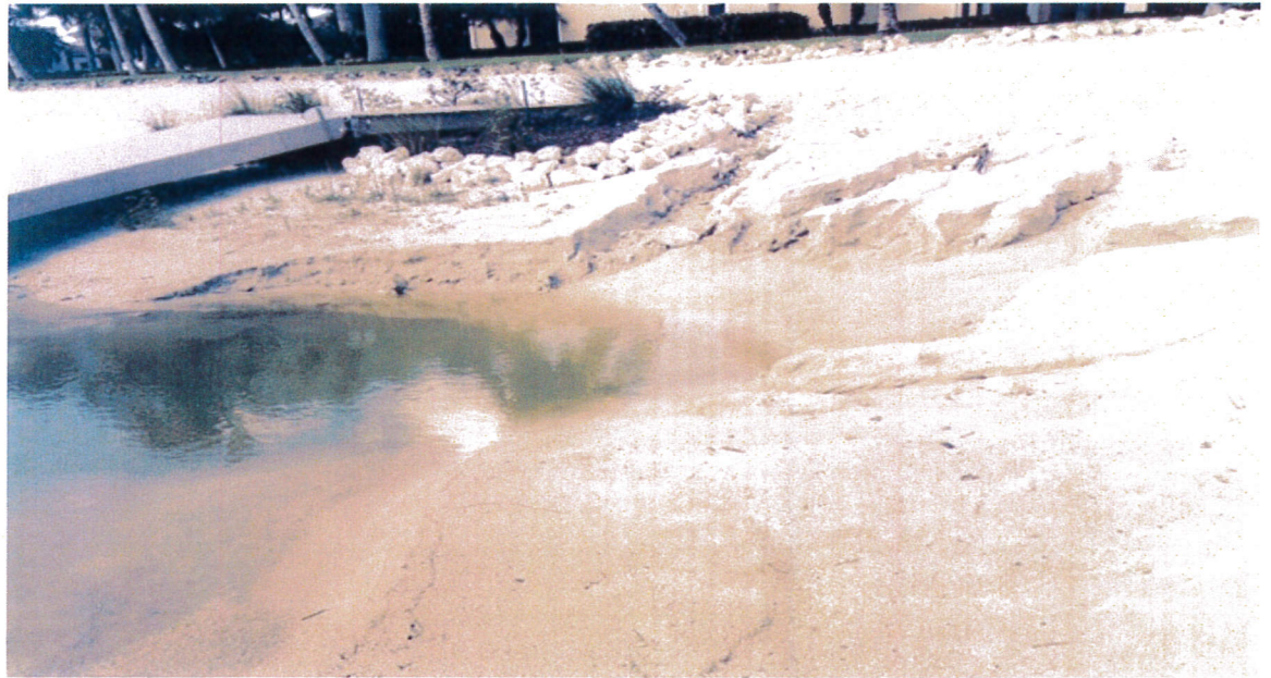
Erosion from drainage outfall after cleaning procedure on beach at Lake 6
