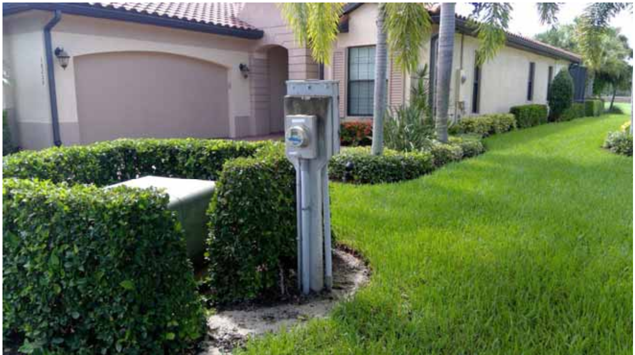
Electrical - Lake Fountain
