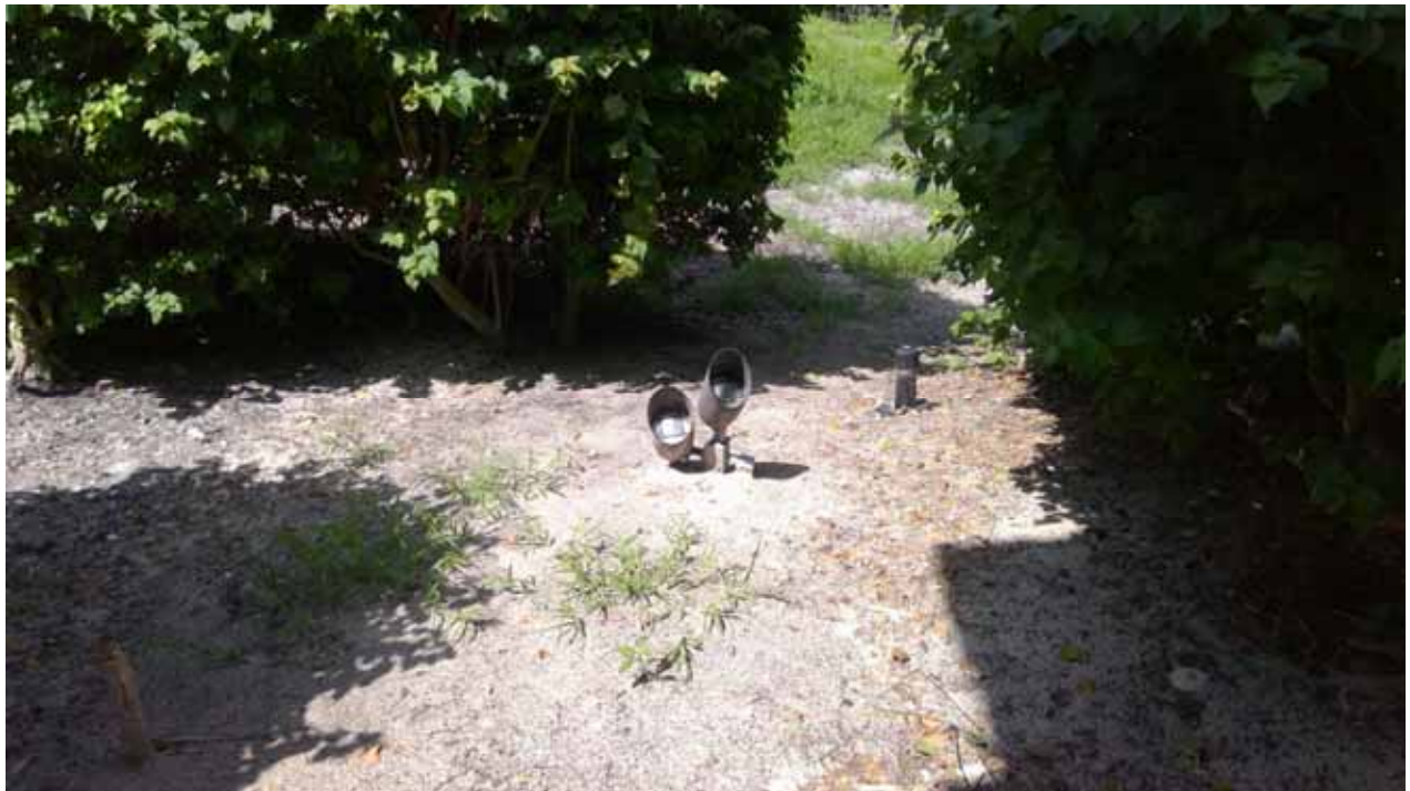
Lighting - Monument I75 South
