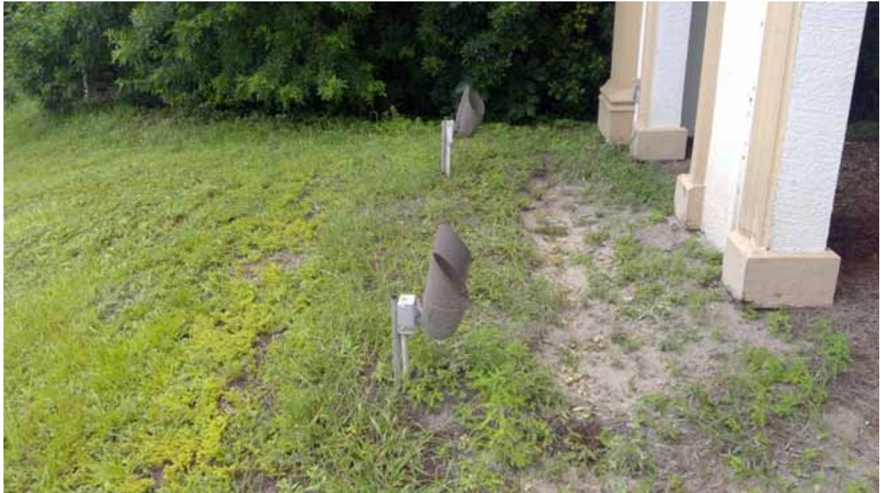
Lighting - Monument I75 North
