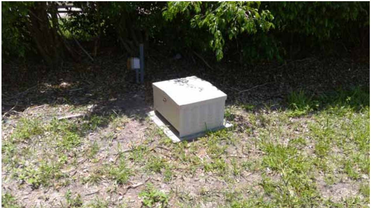
Lake Aerator 1C
