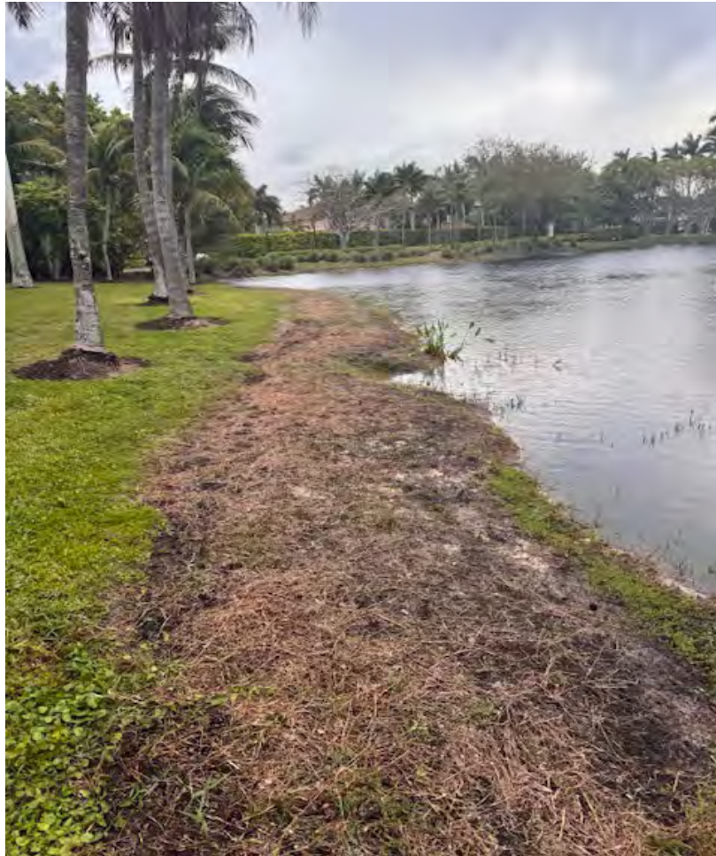
Erosion control needed – Lake 6J
