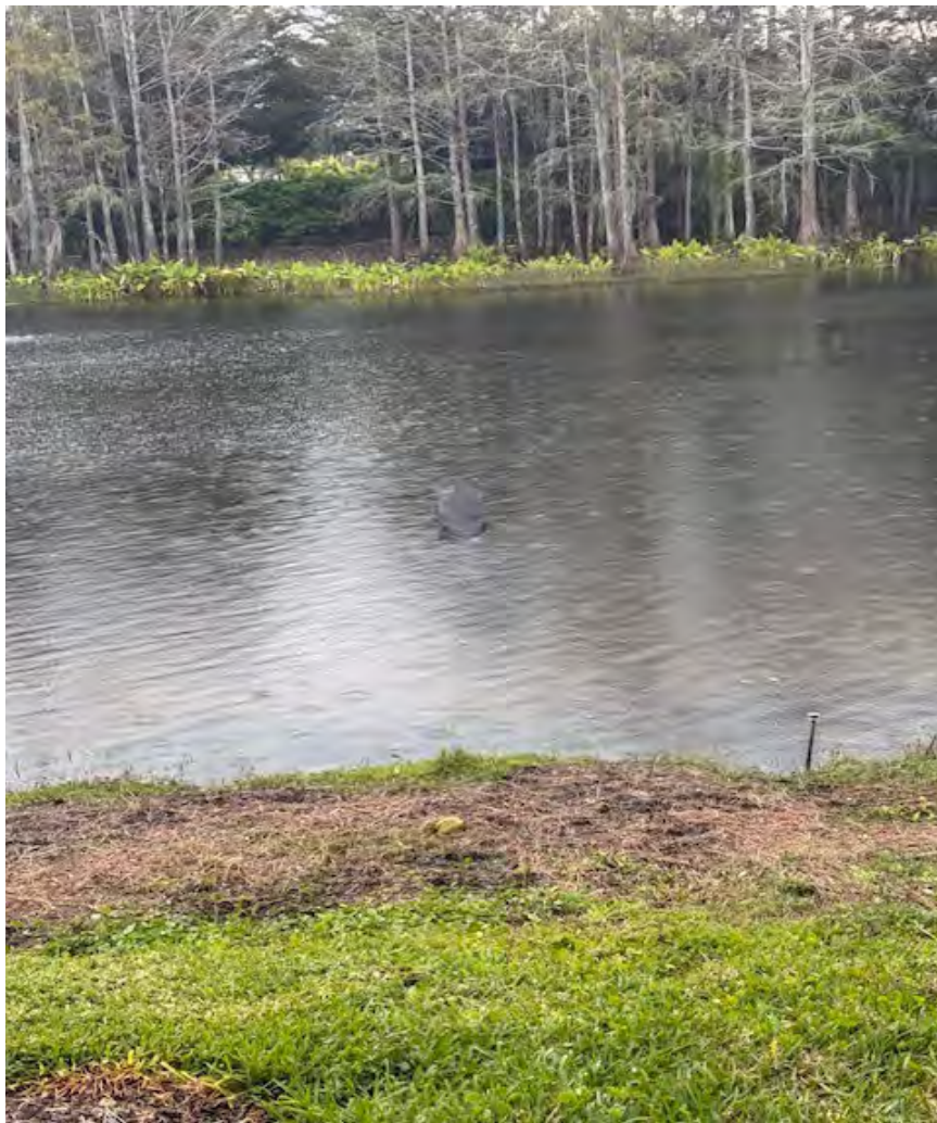
Exposed pipe in Lake 6J
