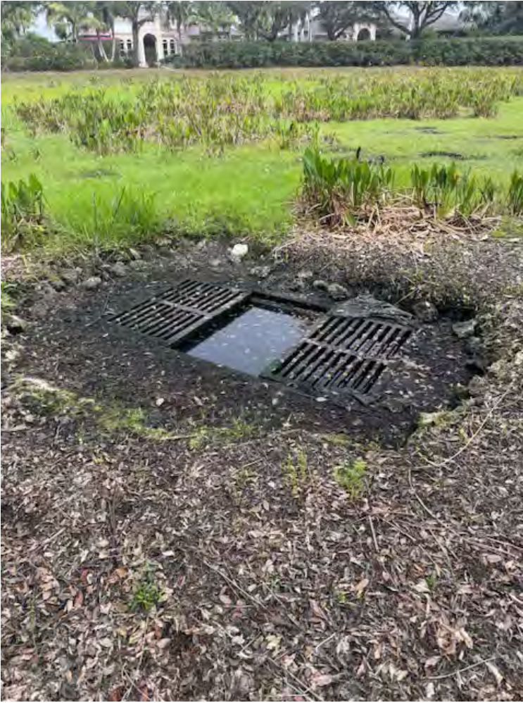
Grate missing in retention area near Verona Logo Drive.
