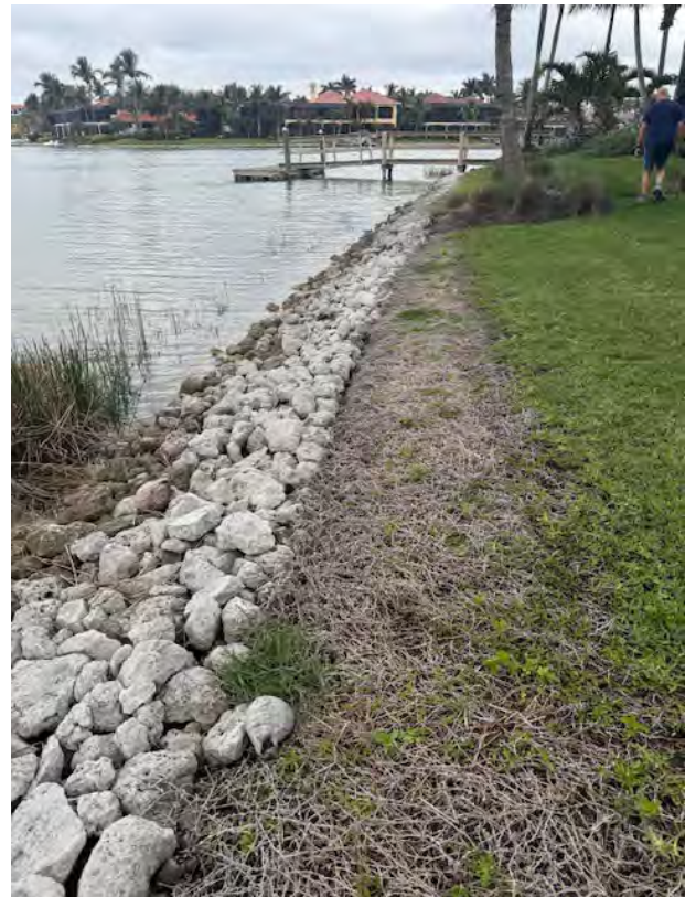
Rip Rap locations needing addition Rip Rap.
