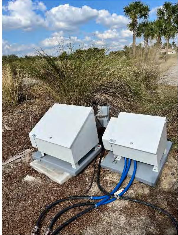
New cabinets for the aeration system.
