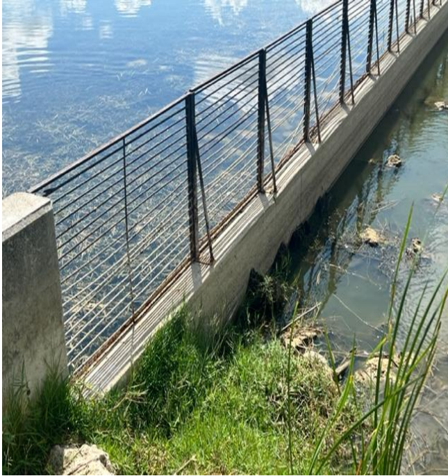
Weir Fence that is Deteriorating
