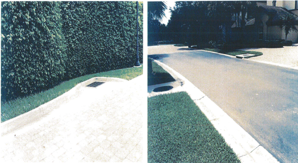
Residential drainage structures for stormwater run-off
