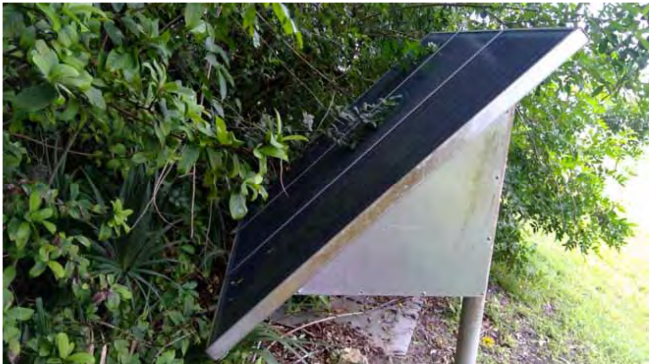
Solar - Monument I75 North
