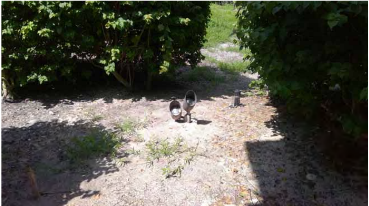
Lighting - Monument I75 South
