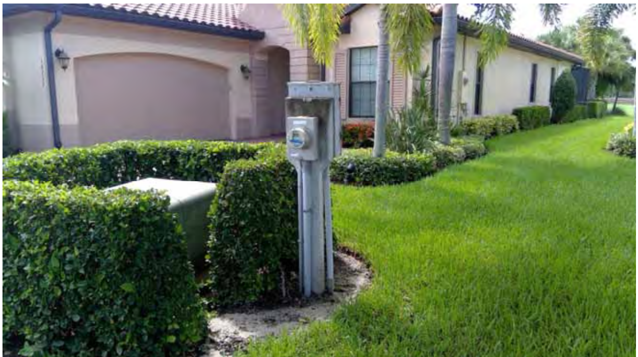
Electrical - Lake Fountain
