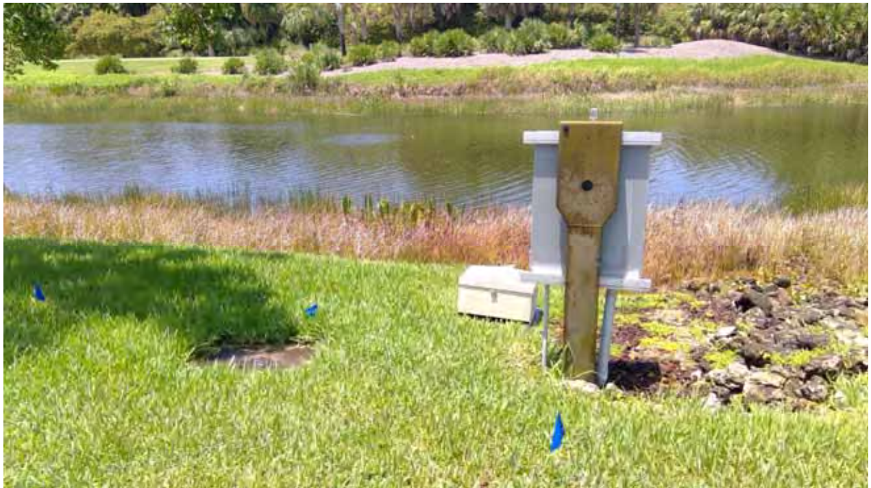
Lake Aerator 1B North
