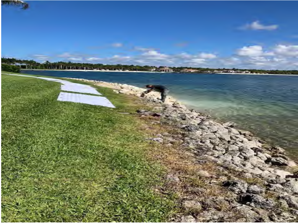
Rib rap installation in progress, with protective materials placed to safeguard surrounding landscaping
