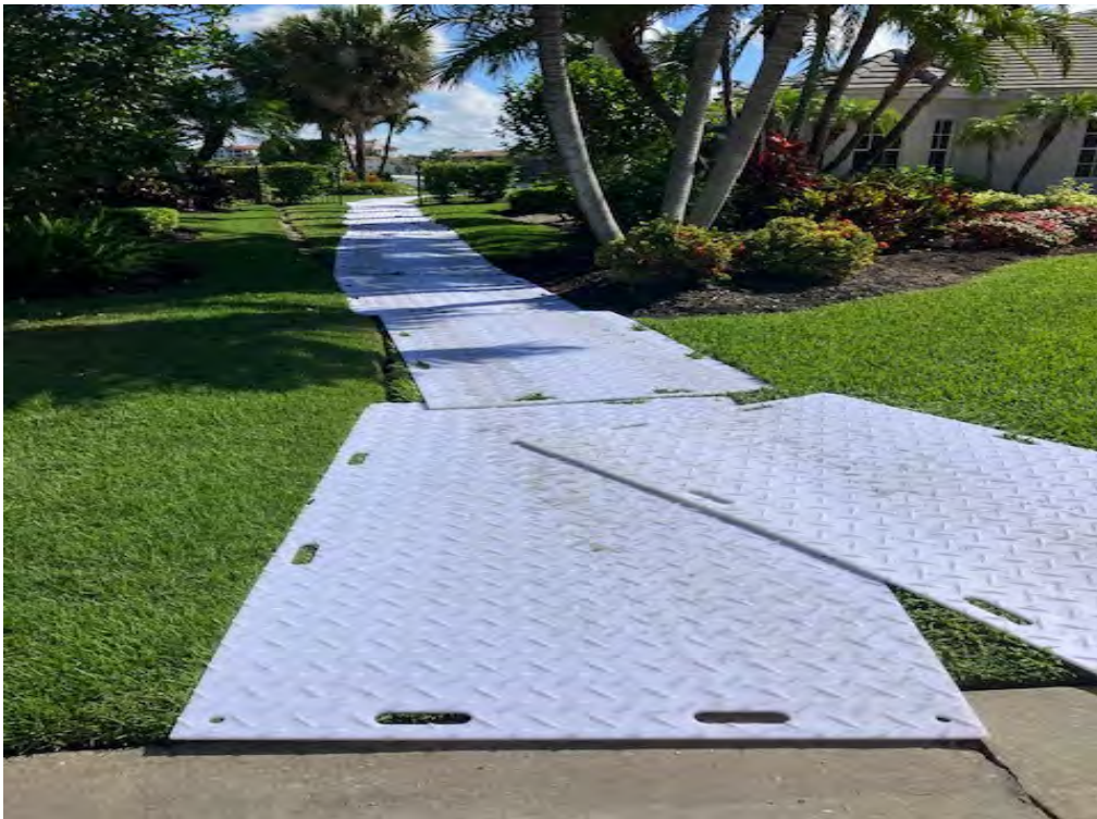
Rib rap installation in progress, with protective materials placed to safeguard surrounding landscaping
