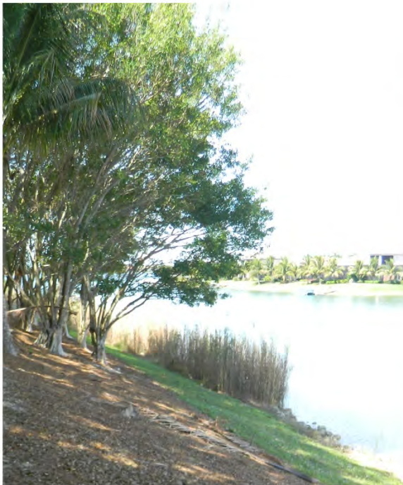
#17 Missing Plants/ Bare Area
