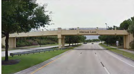
Existing guardrail in median does not provide the same level of architectural treatment as the bridge elements.
