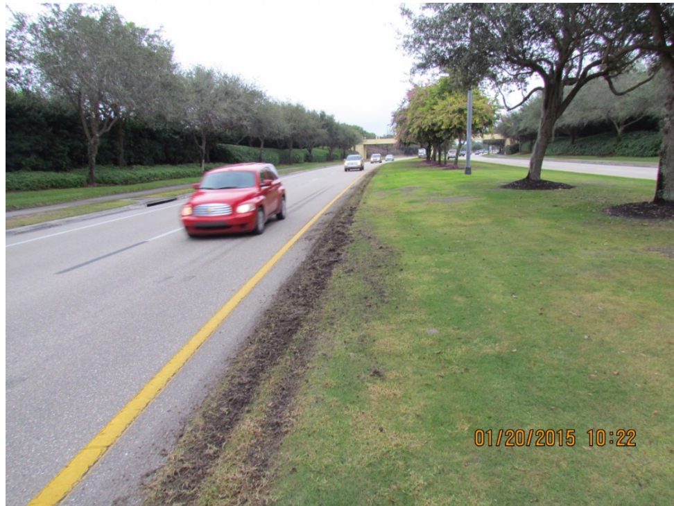
Figure 8- Damage by truck and vehicular traffic in Ben Hill Median
