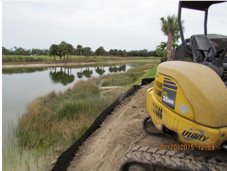
Figure 1- San Marino bank slope under construction by WCI on South Lake Jan. 2015
