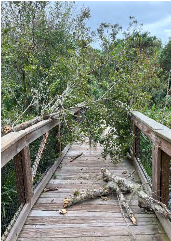
Boardwalk had heavy debris after hurricane.
