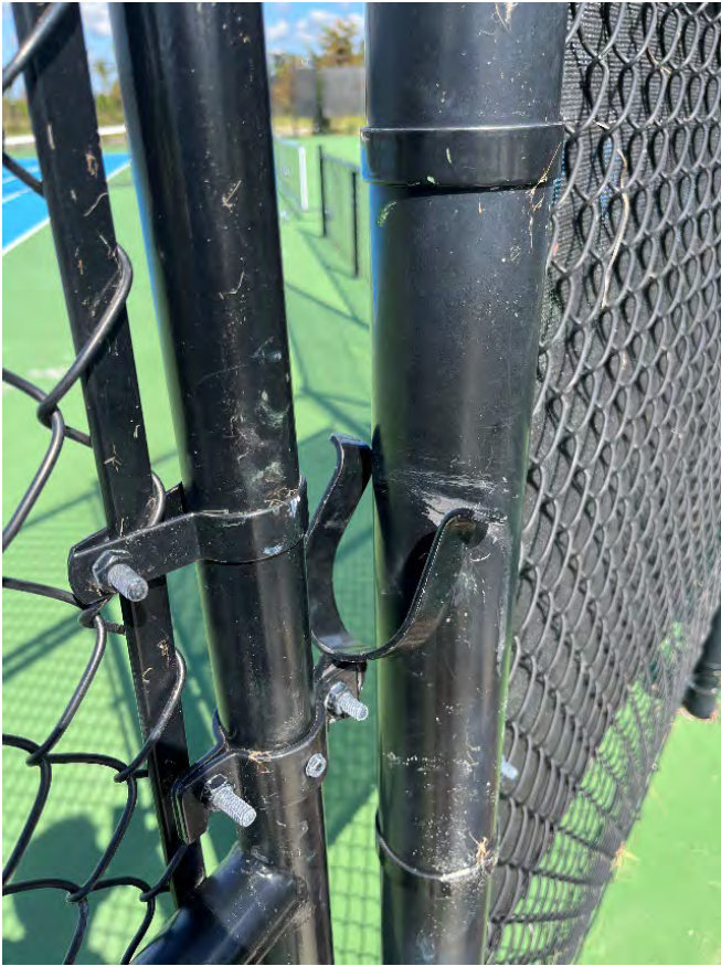
Gate handles on the tennis courts were damaged due to heavy winds.
