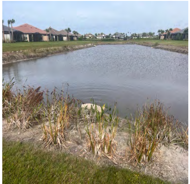
Wash out in L-1 Lake in Esplanade area.
