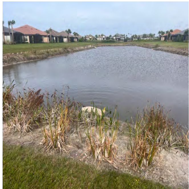
Wash out in L-1 Lake in Esplanade area.
