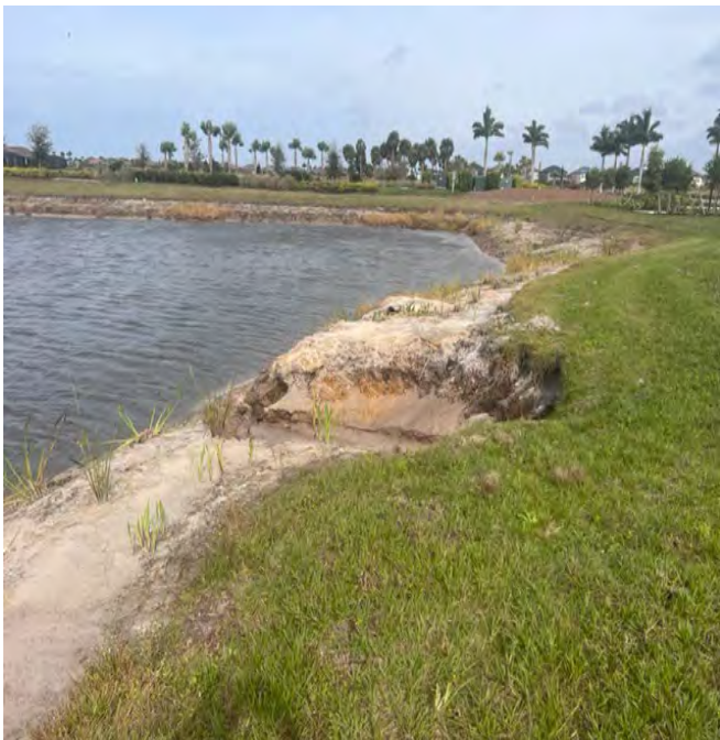
Wash out in J-Lake in Esplanade area.
