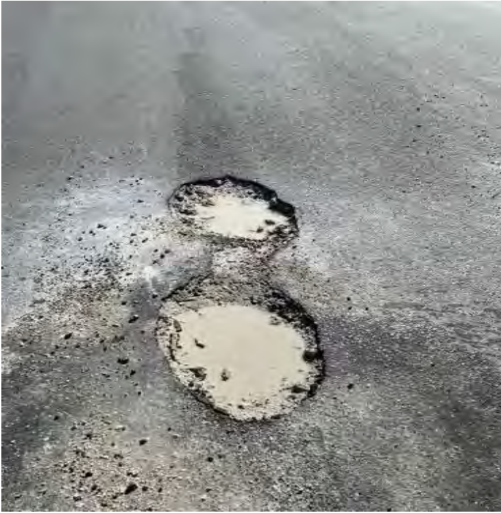
Pothole on Luna Lane that will be replaced in March.
