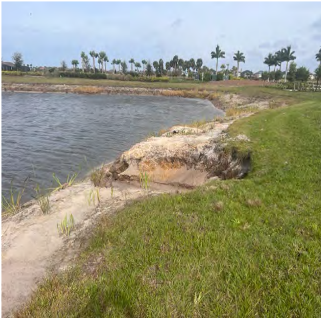
Wash out in J-Lake in Esplanade area.
