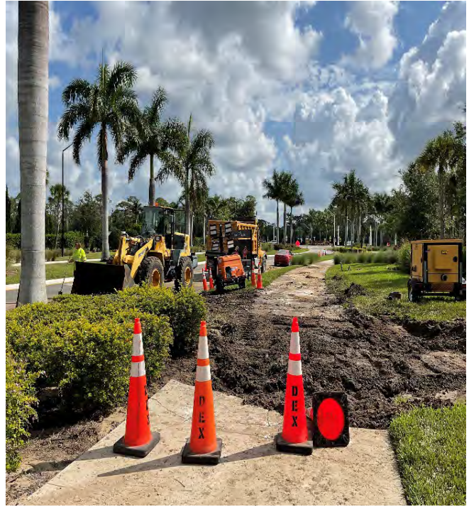
Water main Break
