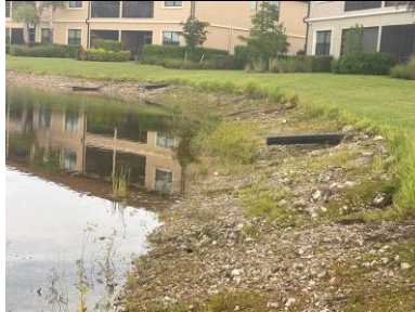
Washout and escarment along homeowner side
