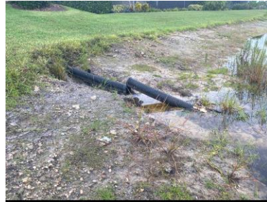
Drainage pipe broke causing washout
