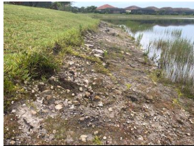
Washout found during inspection
