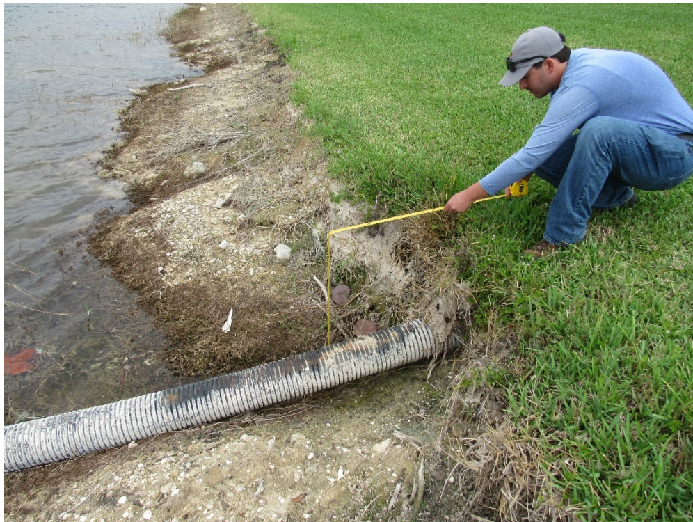
View of the depth of erosion at lake embankment - Lake 20.
