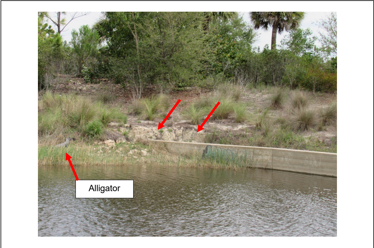
View of erosion - South Broad Crested Weir.
