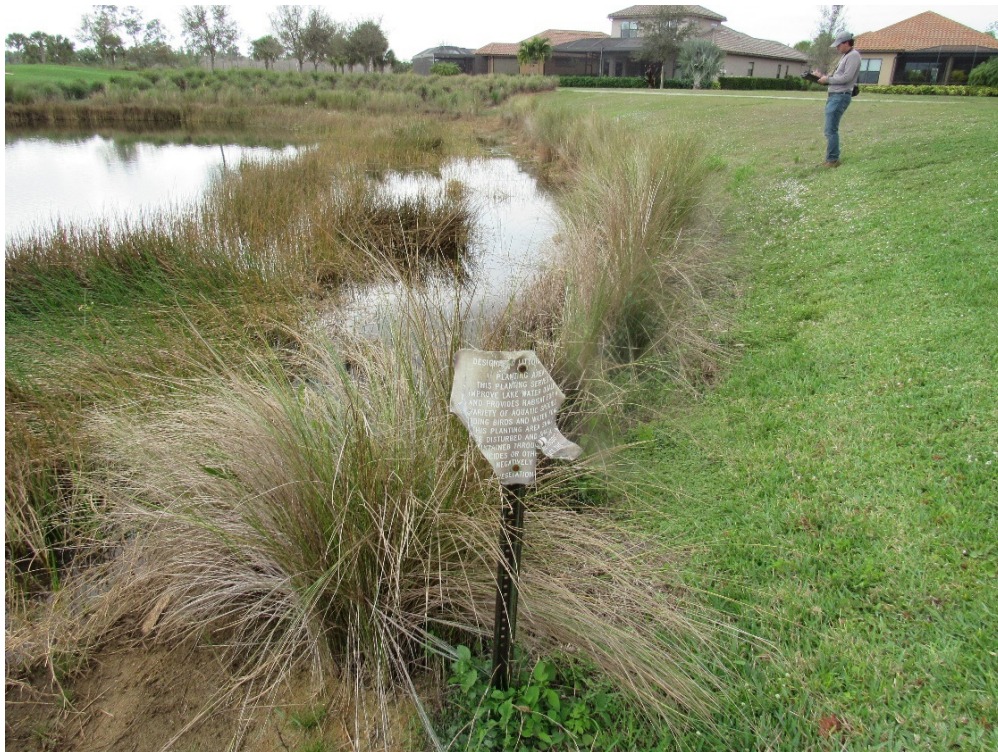
View of damaged Littoral sign - Lake 5B.
