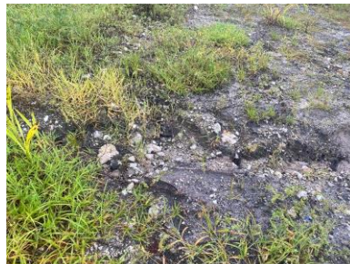
small washout starting
