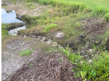
Large washout in corner of lake
