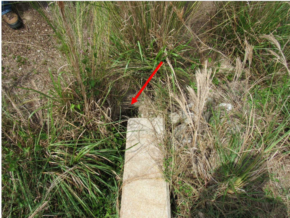
View of erosion - South Broad Crested Weir.
