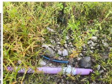
Sprinkler laying down causing washout
