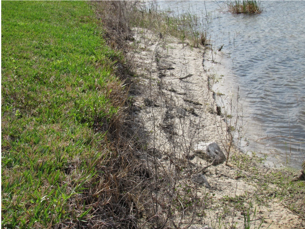
View of erosion at lake embankment - Lake 23.
