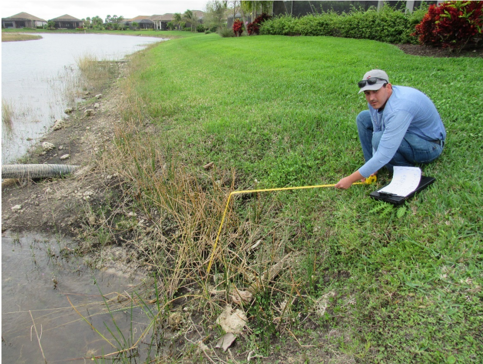
View of erosion at lake embankment - Lake 18.
