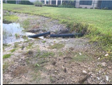
different angle of disconnected pipe
