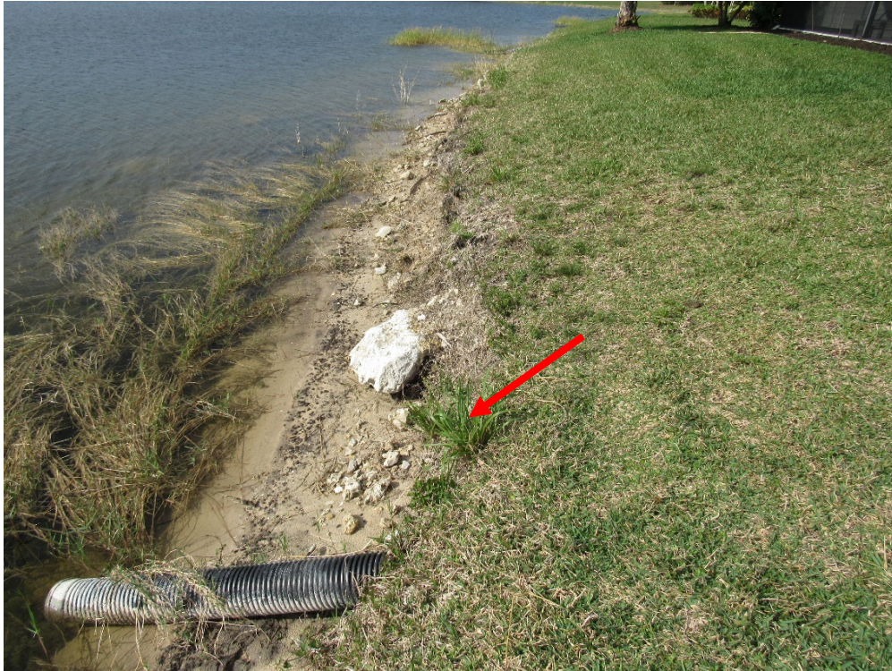
View of erosion at lake embankment - Lake 7.
