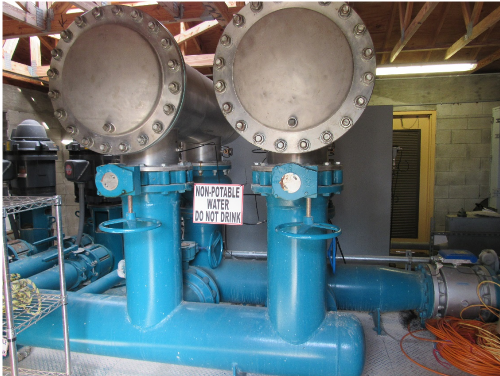
Interior view of Community Irrigation Pump House.
