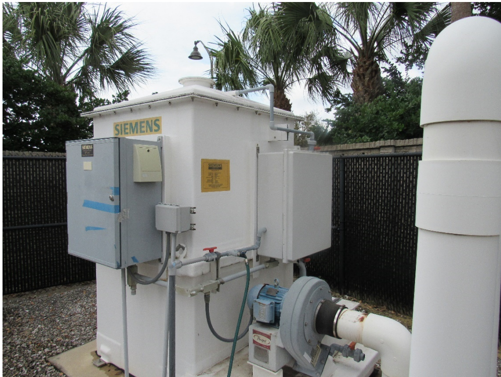
View of odor control system at 168.09.
