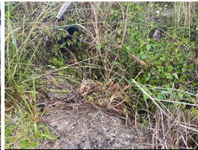
Drainage pipe causing washout
