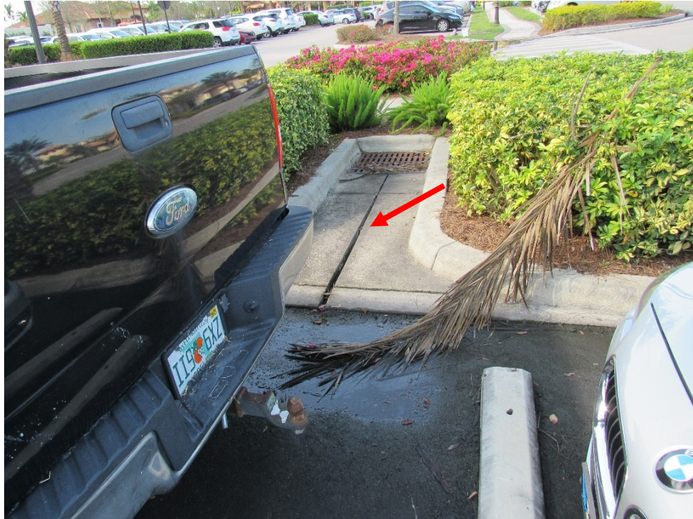
View of groove cut into concrete catch basin – Amenity Center Parking Lot.
