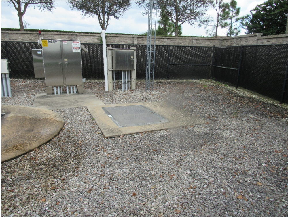
View of lift station 168.09.
