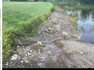
Samll washout starting no plants
