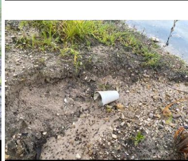
trash found in washout
