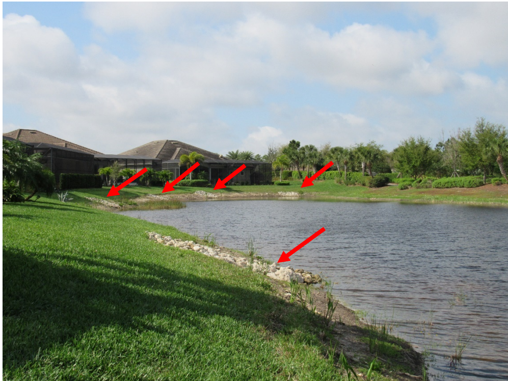
View of rip rap at areas of erosion - Lake 12.
