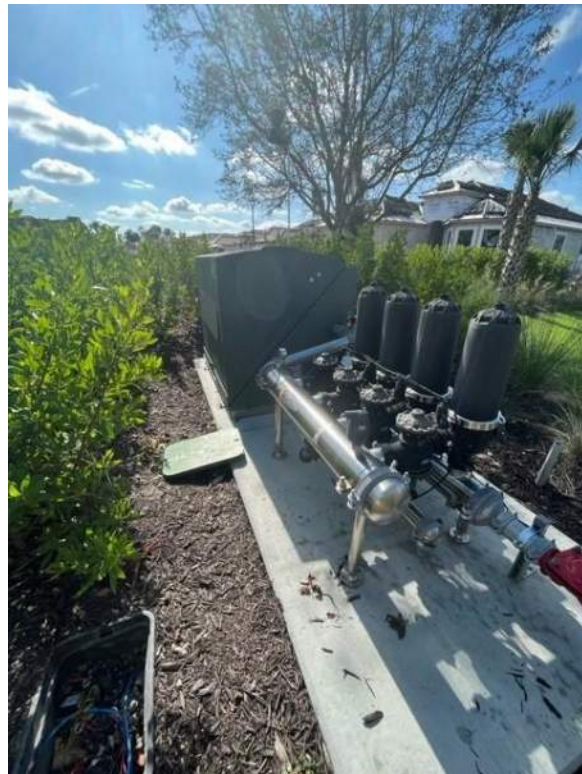
Irrigation - Pumps - Hatcher Parcel
