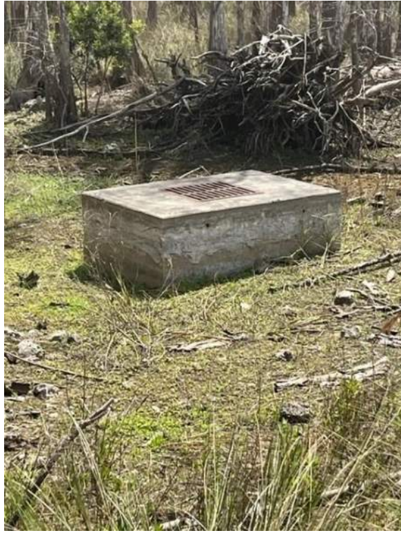
SWM – Bubble-Up Structure
