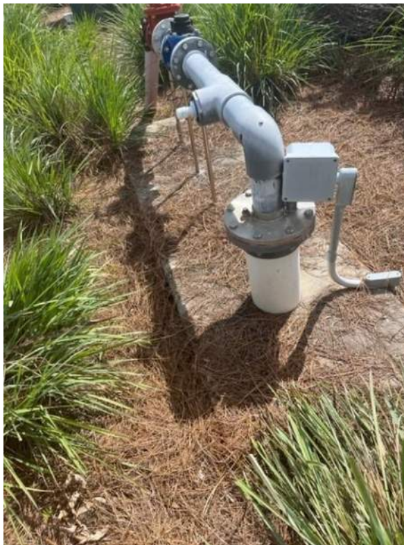
Irrigation - Recharge Well - Hole 12
