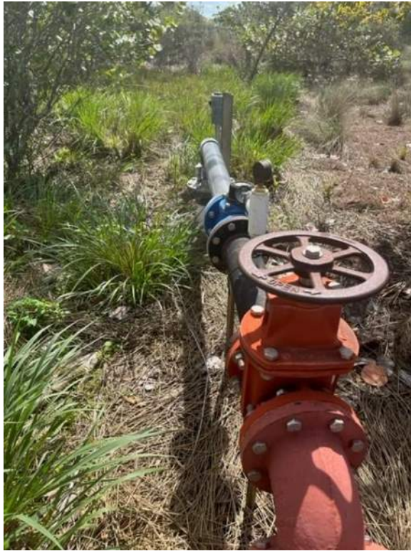
Irrigation - Recharge Well - Hole 11
