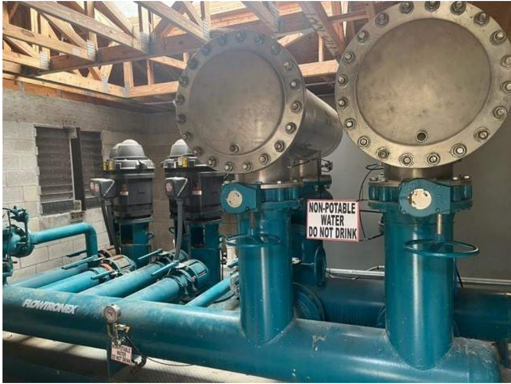
Irrigation - Pump House (Internal)
