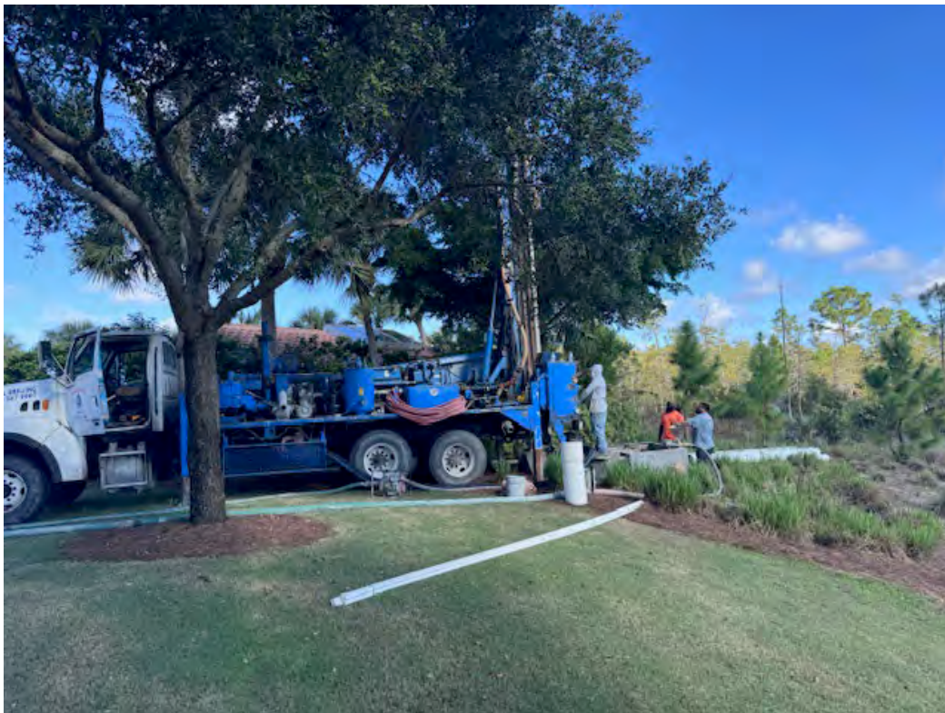
(10) New Emergency Well at Pump House
