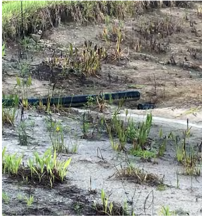
Figure 4-4. Typical condition: displaced piping crossing the shelf directly below residential units, with the surrounding bank stripped of vegetation and the littoral planting failing to establish.
