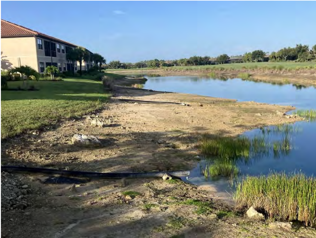
Figure 4-1. Exposed ADS piping daylighted across the lake bank adjacent to residential buildings. The pipe run has no cover and terminates loose on the shelf; note the bare, unvegetated bank and active washout on the near slope.
