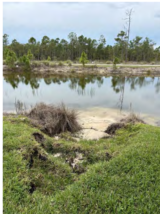
(7) Lake Bank Washout
