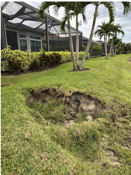
(6) Lake Bank Erosion Behind Residences
