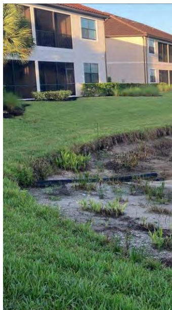
Figure 4-5. Close view of a disconnected joint. The pipe end discharges directly onto bare shelf material rather than at a stabilized outfall point.
