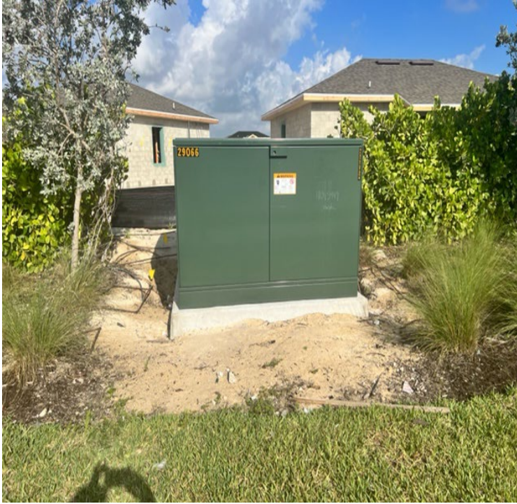
Transformer that was installed on Center Place Blvd.
