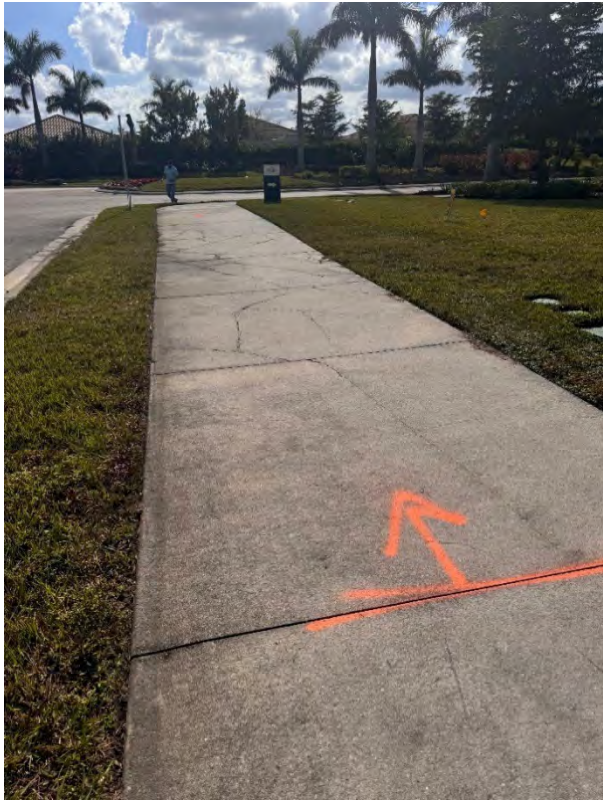
Before the sidewalk was replaced on Center Place Blvd.
