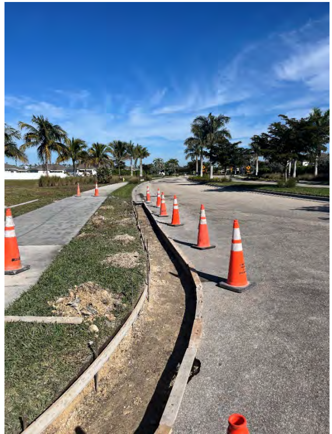
During the replacement for the curb and gutter on Center Place Blvd.
