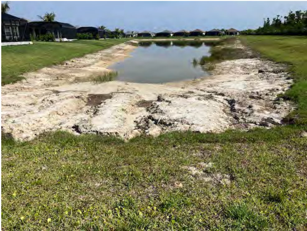
Erosion issues; scheduled installation of littoral plantings
