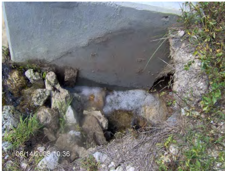
Figure 74: Erosion around the southernmost weir at San Carlos Estates. Source 2008: Exceptional Engineering, Inc.
