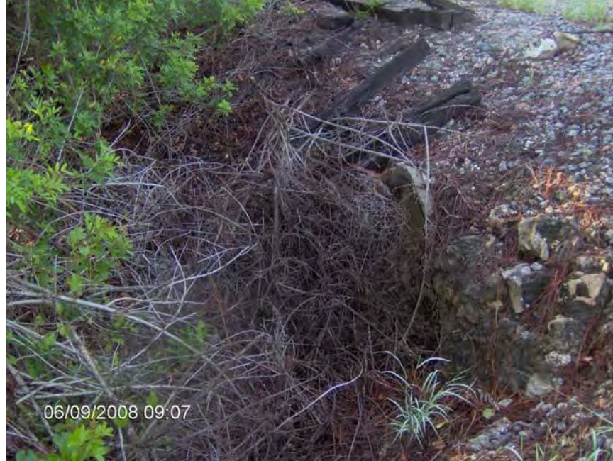
Pic 13. Additional Pipe at Railroad Crossing
