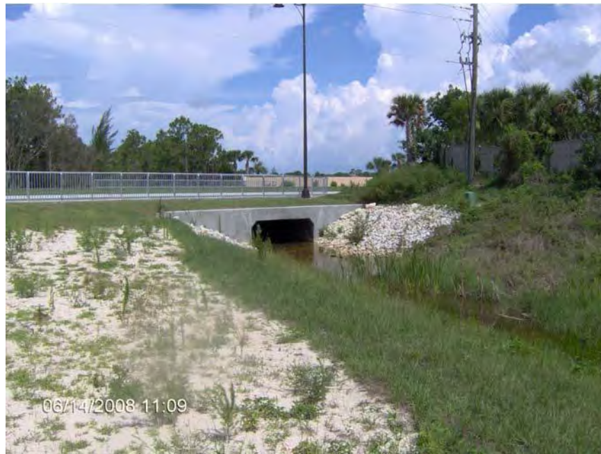
Figure 54: Box Culvert at Three Oaks Parkway Extension east side Source: 2008, Exceptional Engineering, Inc.
