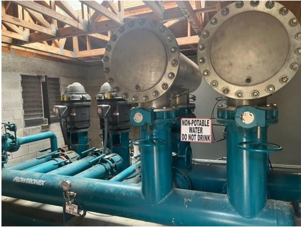
Irrigation - Pump House (Internal)
