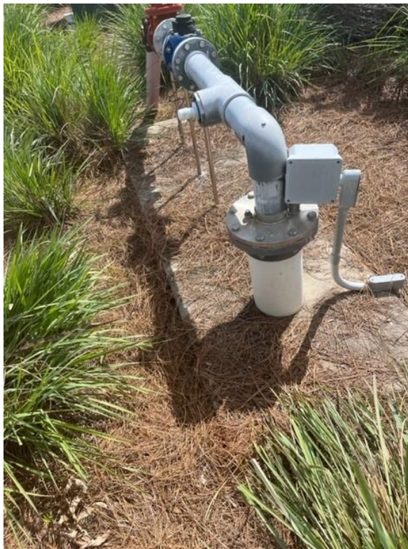
Irrigation - Recharge Well - Hole 12
