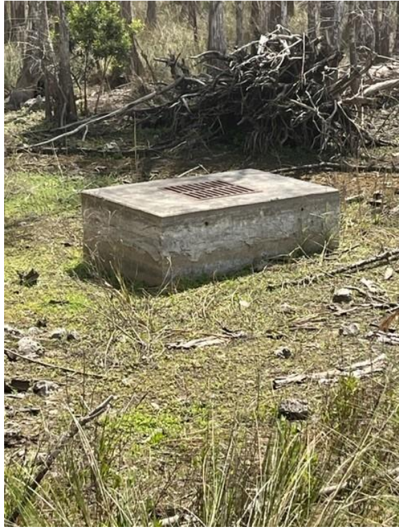
SWM – Bubble-Up Structure
