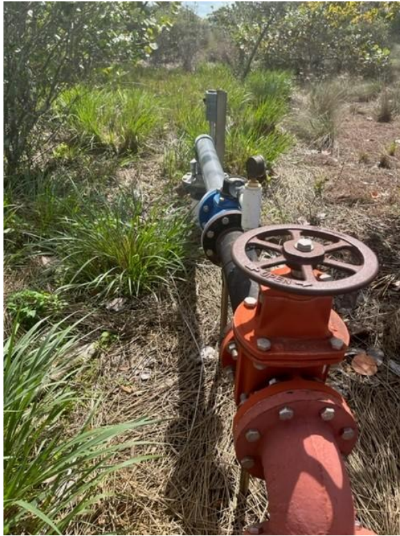
Irrigation - Recharge Well - Hole 11
