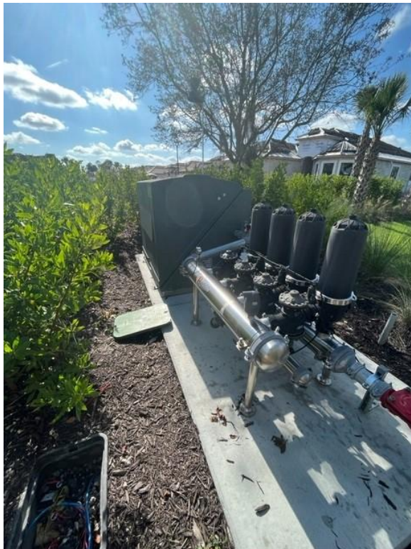
Irrigation - Pumps - Hatcher Parcel
