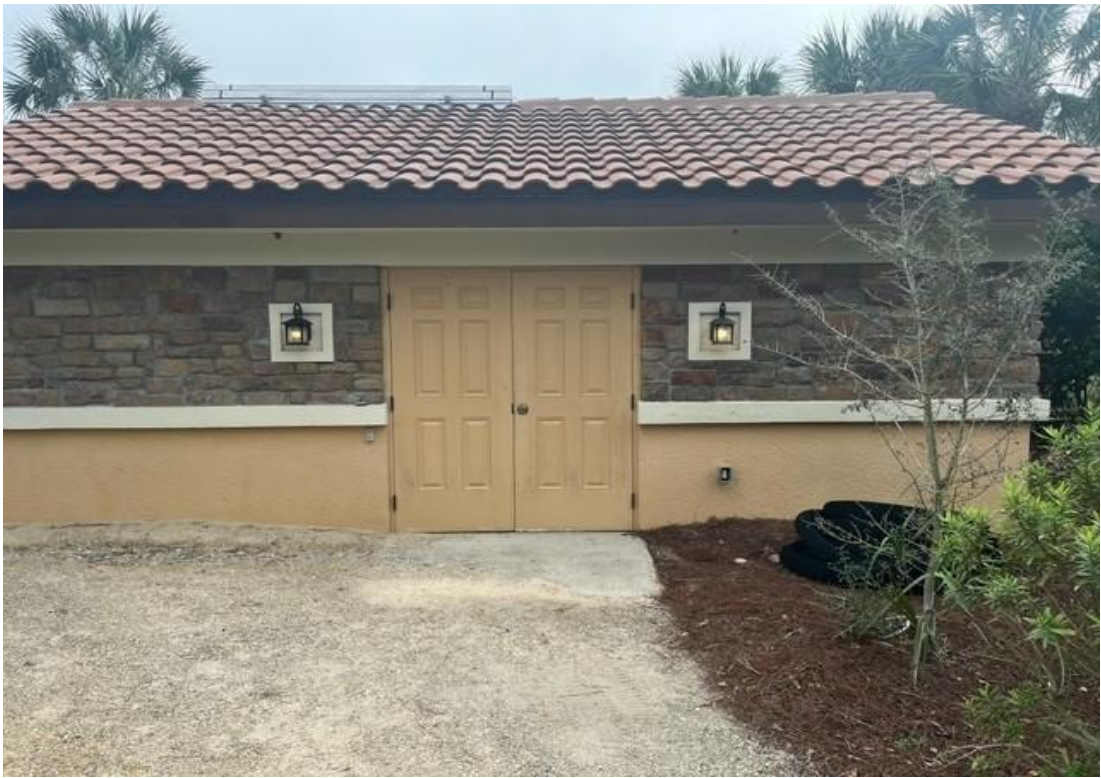
Irrigation - Pump House (External)
