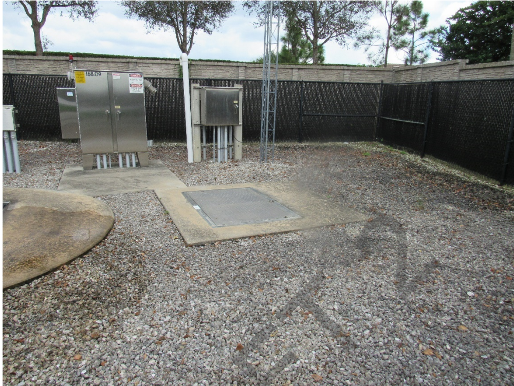
View of lift station 168.09.
