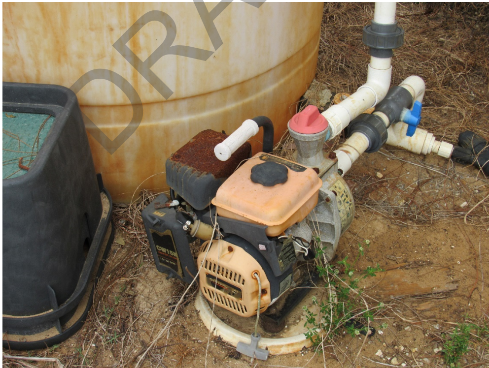
View of exterior gas pump - Golf Course Irrigation Pump House.
