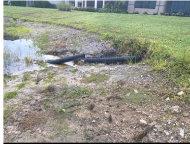
different angle of disconnected pipe
