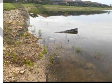
Pipe not anchored down
