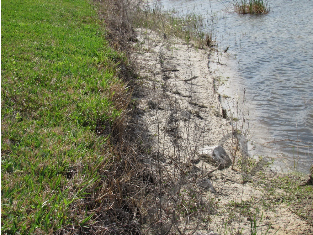
View of erosion at lake embankment - Lake 23.
