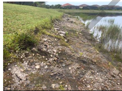
Washout found during inspection
