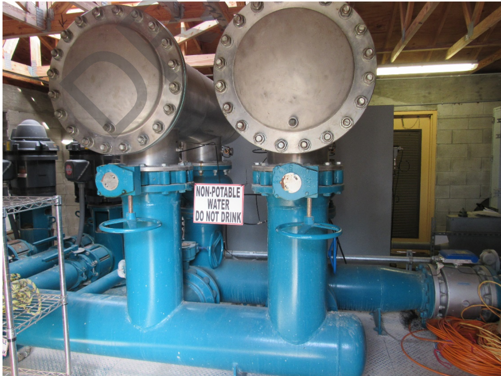
Interior view of Community Irrigation Pump House.
