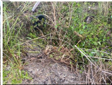
Drainage pipe causing washout
