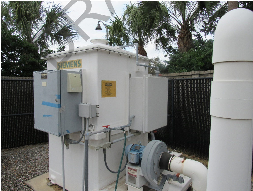
View of odor control system at 168.09.
