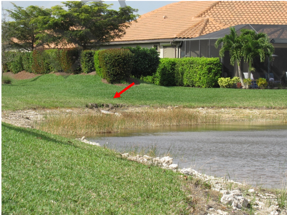
View of erosion at lake embankment - Lake 15A.
