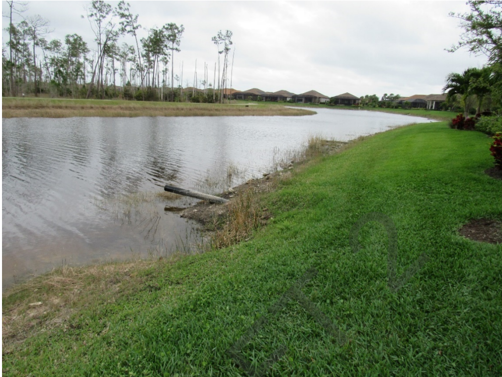
View of erosion at lake embankment - Lake 18.
