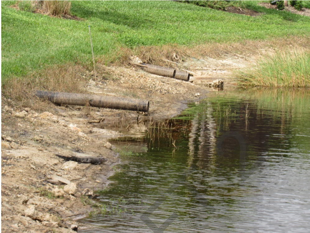
View of erosion at lake embankment and direct discharge lines - Lake 16.
