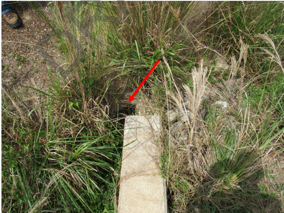
View of erosion - South Broad Crested Weir.
