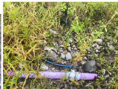
Sprinkler laying down causing washout
