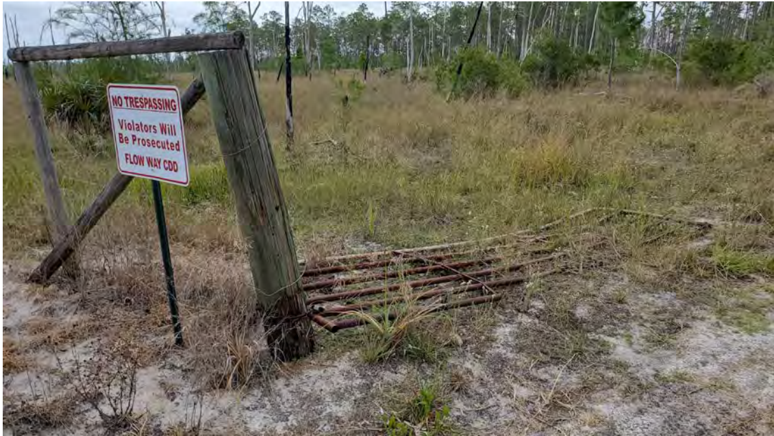
#46 - Flow Way CDD Gate 1 – Broken
