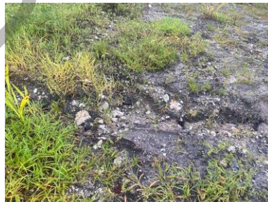
small washout starting
