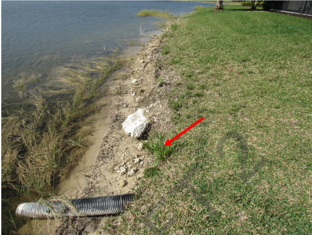
View of erosion at lake embankment - Lake 7.
