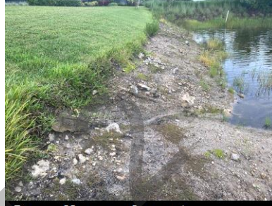
Small washout starting no plants
