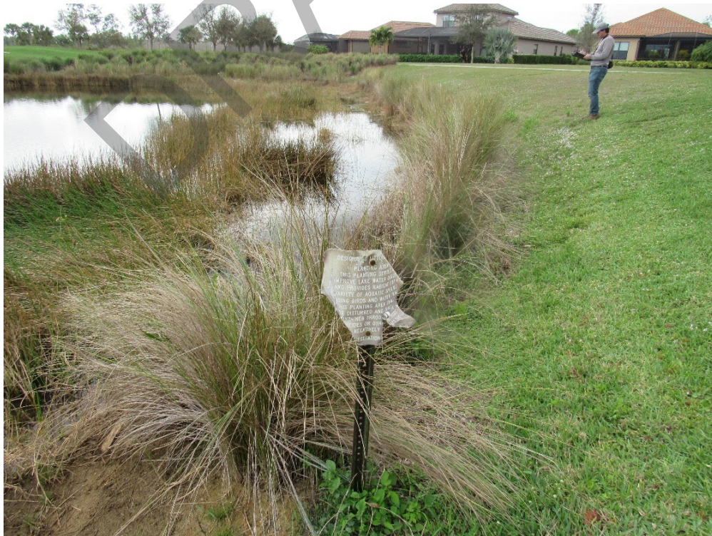
View of damaged Littoral sign - Lake 5B.
