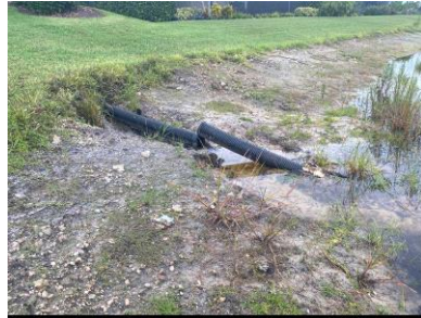
Drainage pipe broke causing washout
