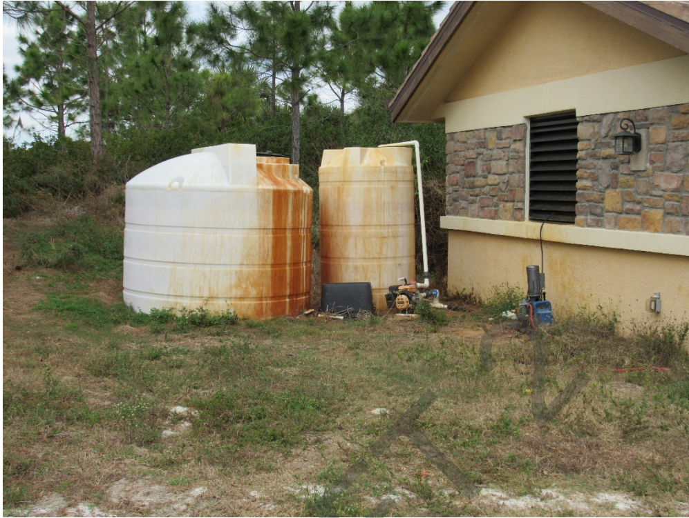
View of unknown tanks - Golf Course Irrigation Pump House.
