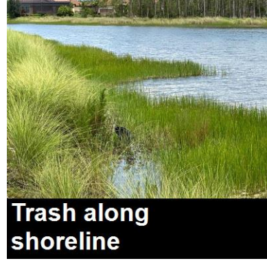
There is new erosion present at the time of inspection.
