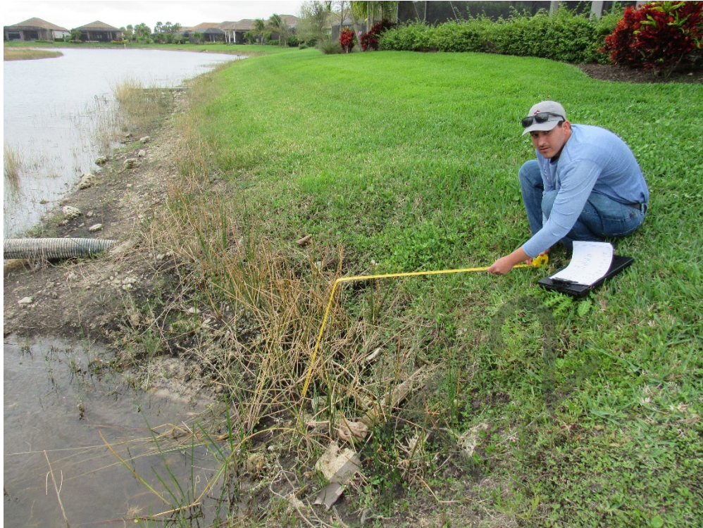
View of erosion at lake embankment - Lake 18.
