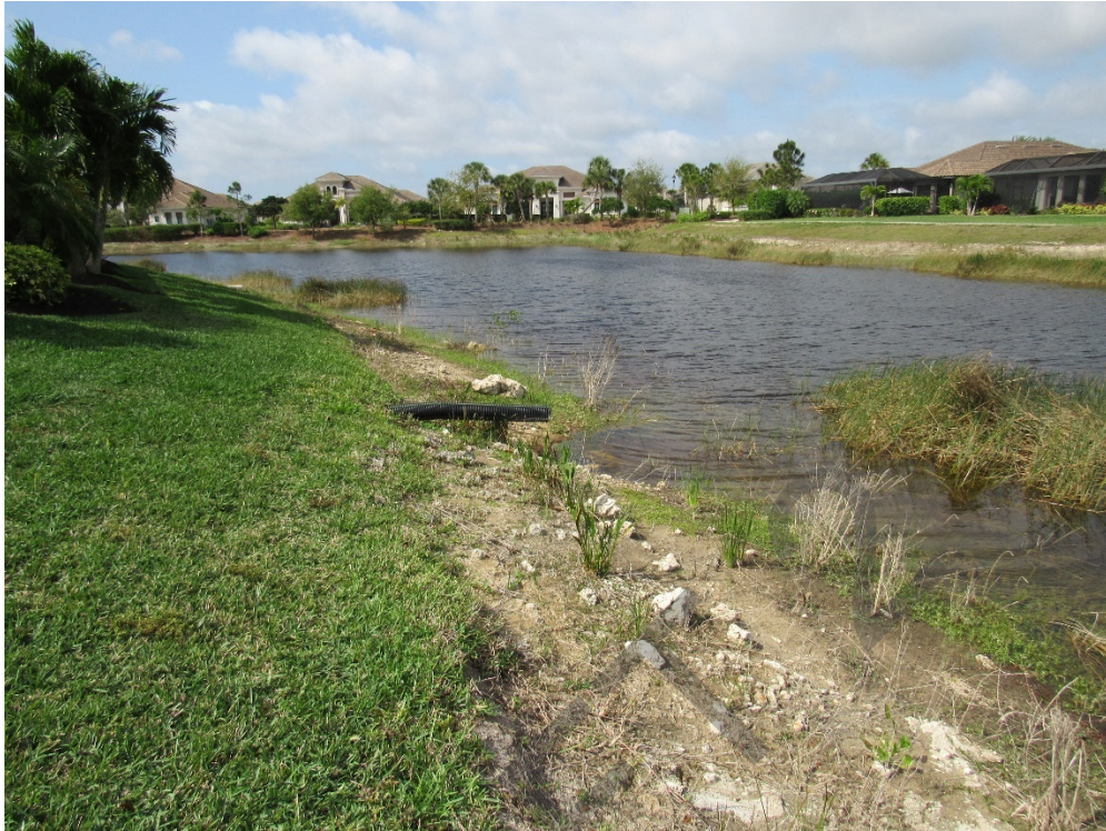
View of erosion at discharge line - Lake 14.
