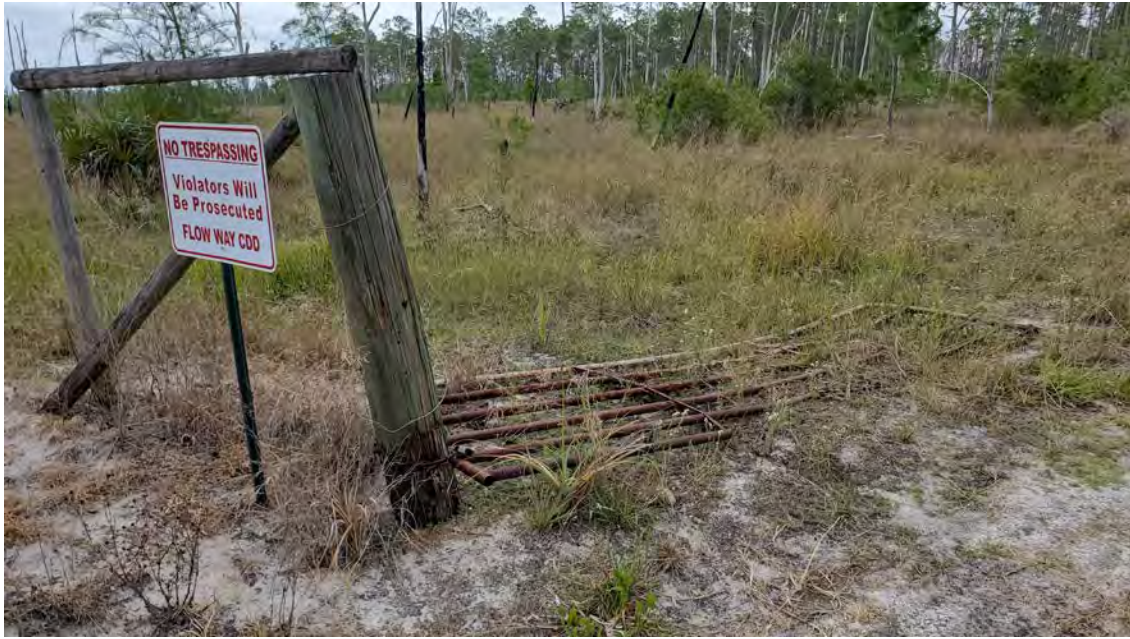
Flow Way CDD Gate 1 – Broken
