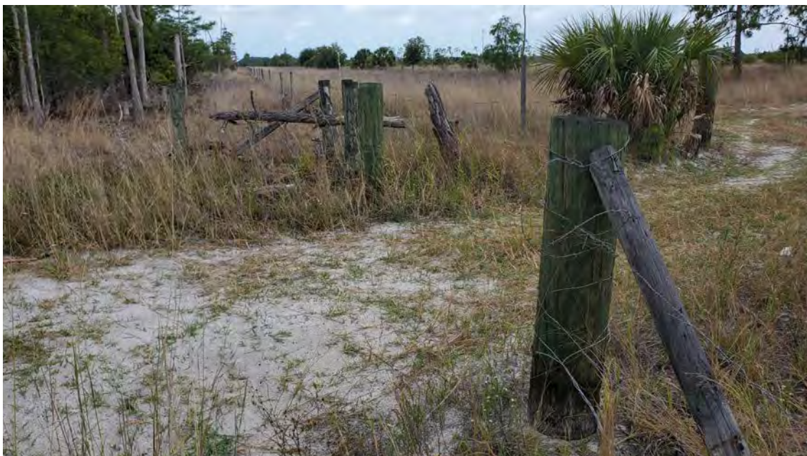
#51 - Flow Way CDD Gate 2 – Broken
