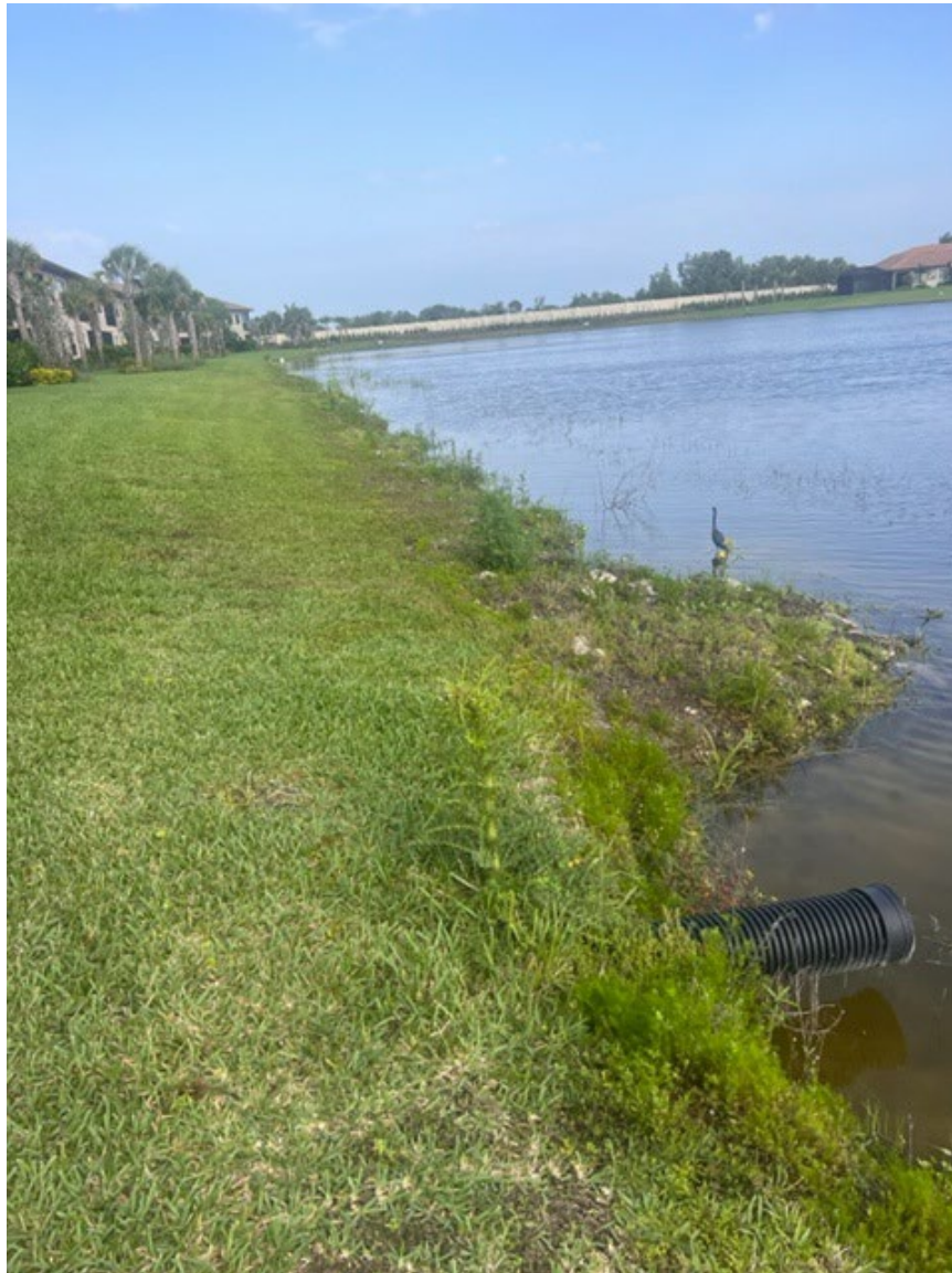
Erosion issues on Lake E1.
