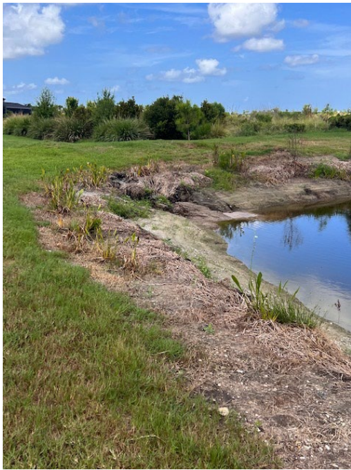
Hog damage on Lorrain Blvd.
