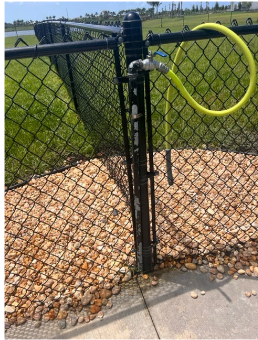
Hog damage on Lorrain Blvd.
