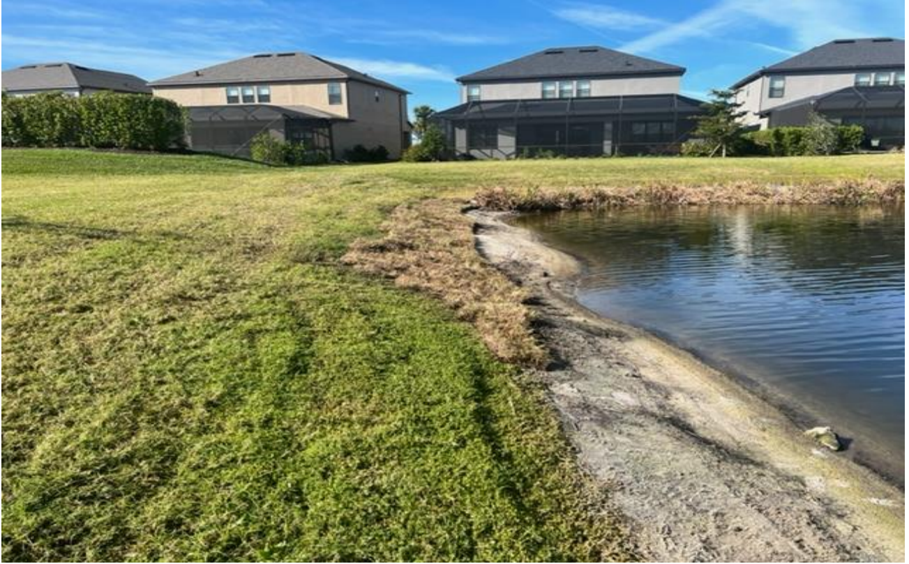
Washout Repair That Was Made on Lake H2
