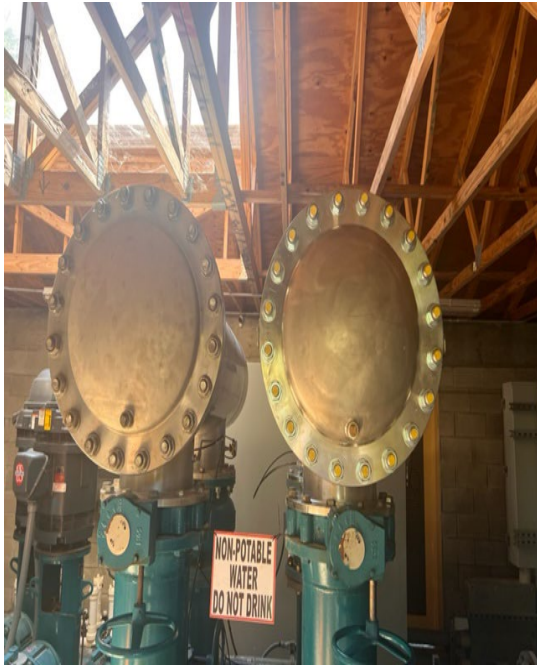
New canister filter in the pump house.
