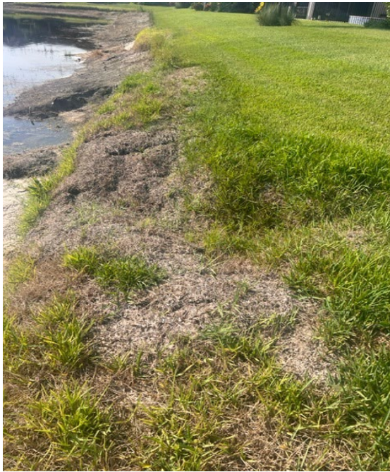
Washout behind residential homes need to be repaired. Covered under warranty.
