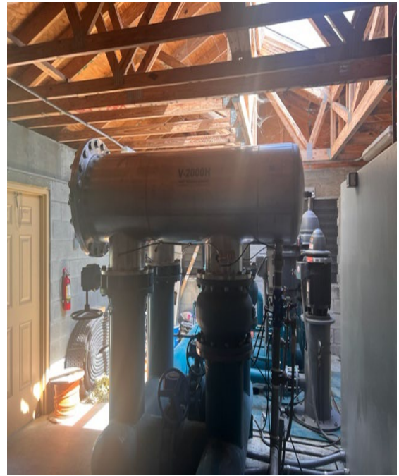
New canister filter in the pump house.
