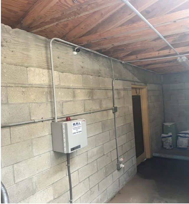
Camera installation in the pump house.
