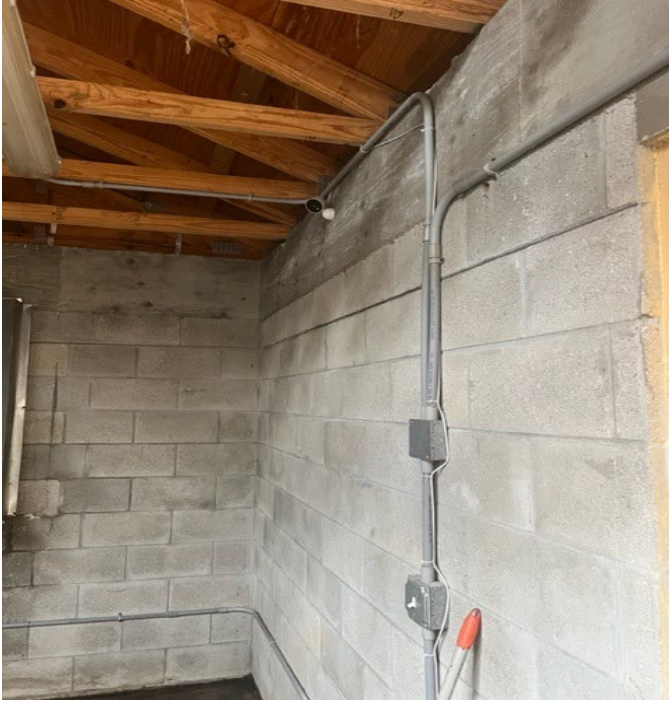
Camera installation in the pump house.
