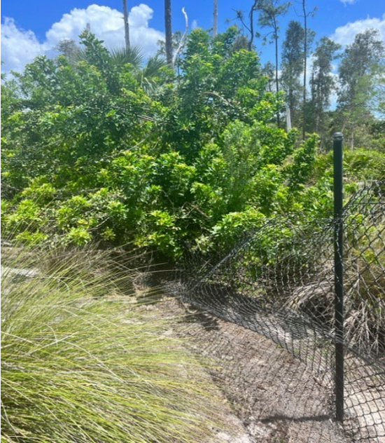
Perimeter fence damage at Nature Trail.
