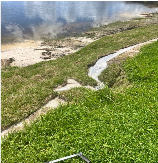
Lake Bank erosion post-construction.
